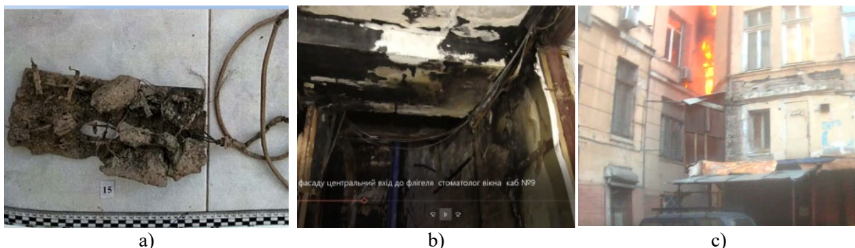
Fig. 1. Consequences of the emergency mode of operation of the electric extension cord:
