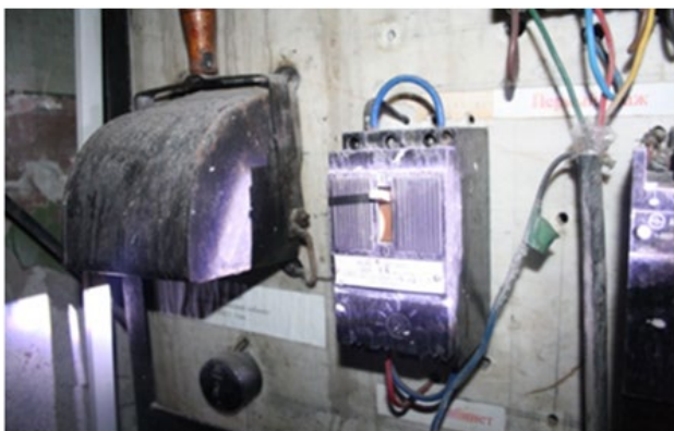
Fig. 2. Photo of an automatic switch with shunt jumpers of input and output contact groups for phases "A" and "C".
