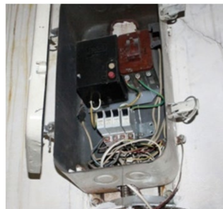
Fig. 3. Photo of an automatic switch with shunt jumpers of input and output contact groups for phases "A" and "B".
